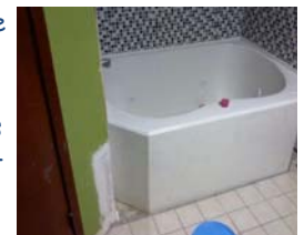
Here is the beautiful new Marathon tub installed, with the new tile work his wife did. He stated that all that is left is to re-paint the surrounding sheetrock.
